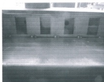
Holes through which the flue gases pass, regulated by the damper of the oven
